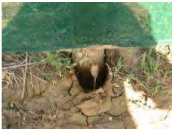
Figure 4.18 Post movement from High wind
