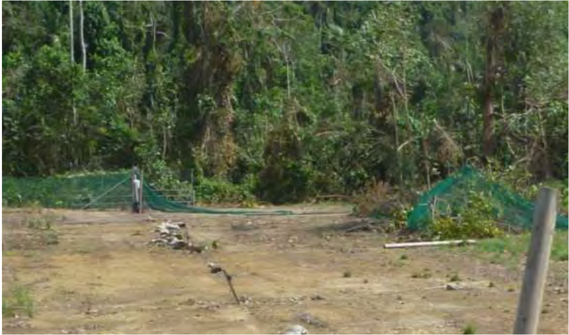
Figure 4.27 Cyclone Yasi 300m fence Northern end. Fence into the vegetation intact and undamaged. The section of fence and posts from the mid-strainer destroyed.
