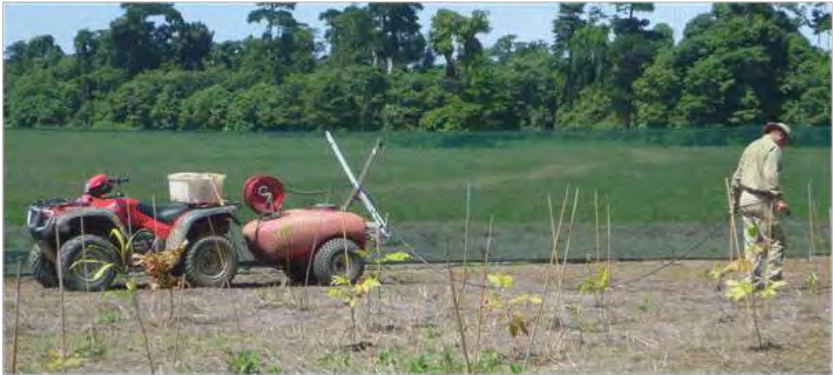
Figure 4:7 North West corner spot spraying prior to fabrication of custom spray boom.
