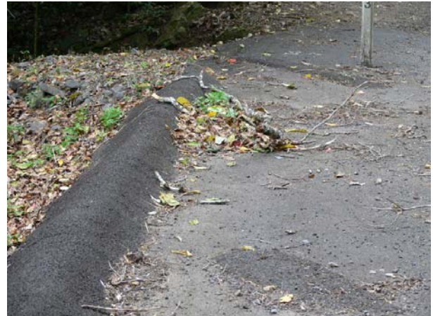
Plate 25. Close-up of a similar hot-mix “kerb” on the Kuranda Range Road (August 2007).
