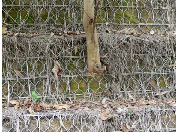
Plate 10. Fallon Road – example of integrity of mesh with tree growing through. It remains to be seen what effect the stiff steel grid will have on the trunk once it is encountered by the growing tree.
